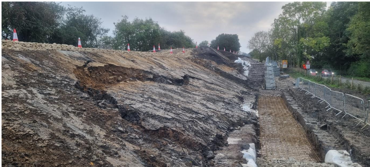
Figure 2 - Slope failure within existing historic embankment during construction works
