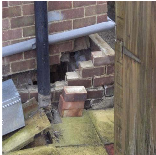
Subsidence at Windsor Drive, Hertford
