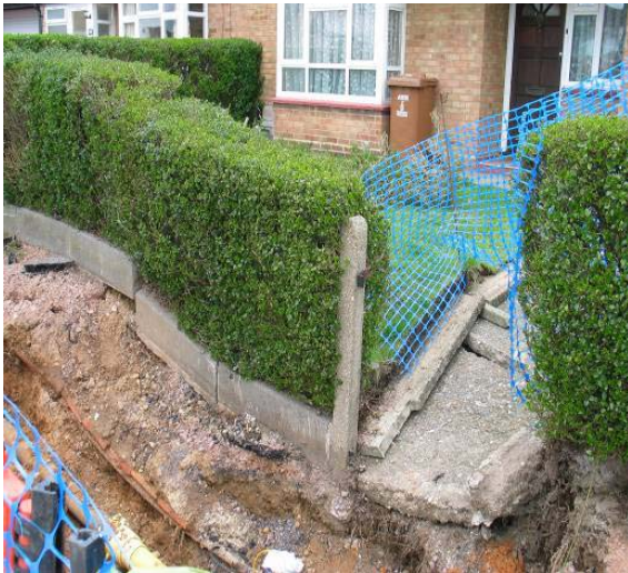
Subsidence at Queens Drive, Rickmansworth
