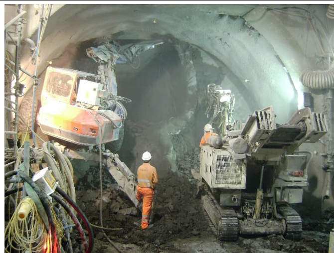
Simultaneous excavation of an enlargement and breakout of a pilot tunnel at King's Cross, 2007.
