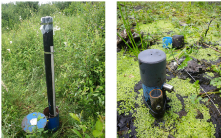
Left to right: Borehole 4 extended with re-enforced PVC tubing to contain artesian groundwater levels; a 'fixed and floating' dipwell pair in a quaking area of the fen, designed to detect the vertical movement of any floating surface raft within the fen.
