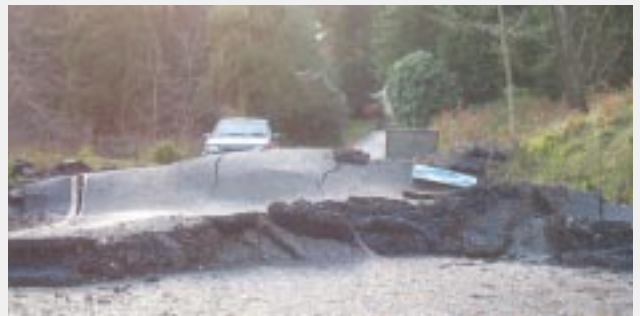
Pictured: Damage to a road caused by the Leith Hill landslip (Surrey), which was reactivated by heavy rainfall in December 2000. Photo: Mike Stephen.
